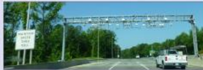
Overhead tolling gantry
